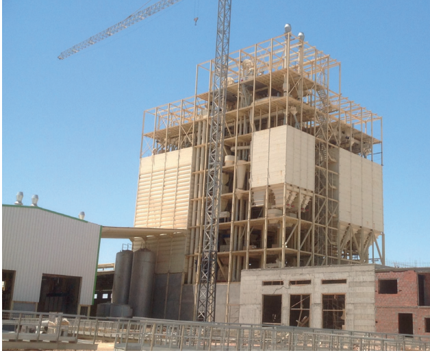
Project: Cattle Feed Factory (Tunisia) Client: Medimix
