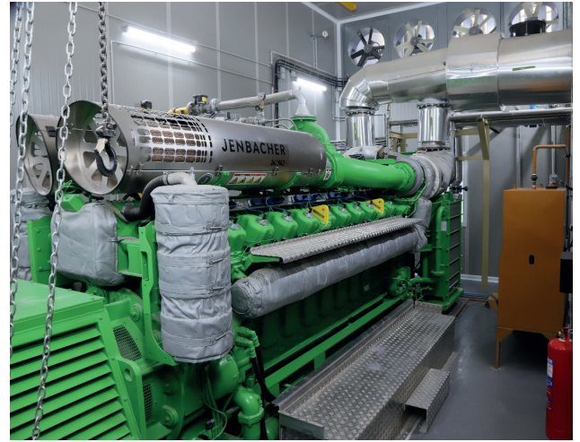
Project: Cogeneration (Sfax - Tunisia) Client: STPA
