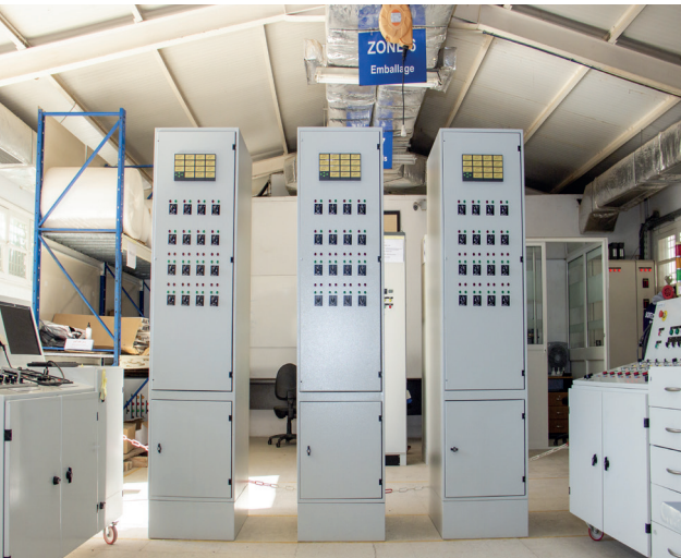
Project: Electrical Panels (Libya) Client: GETS
