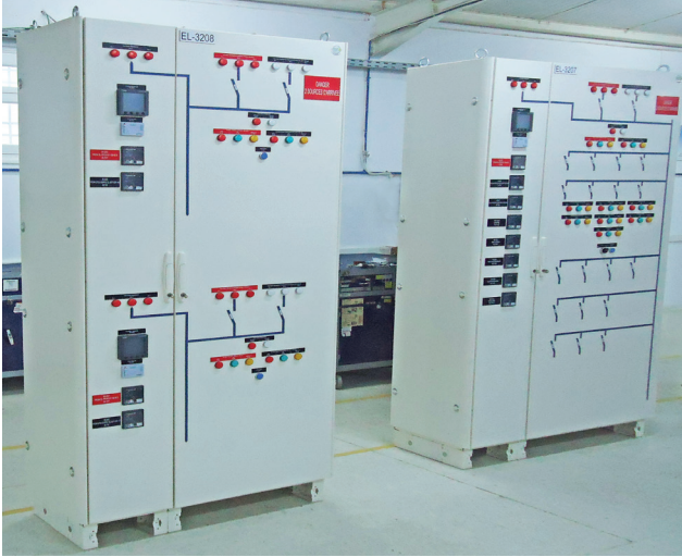
Project: Supply & installation of electrical distribution equipment (Sfax - Tunisia) Client: British Gas
