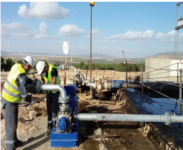
Project: Electrical works in an oil pumping station (Douleb - Tunisia) Client: Serept
