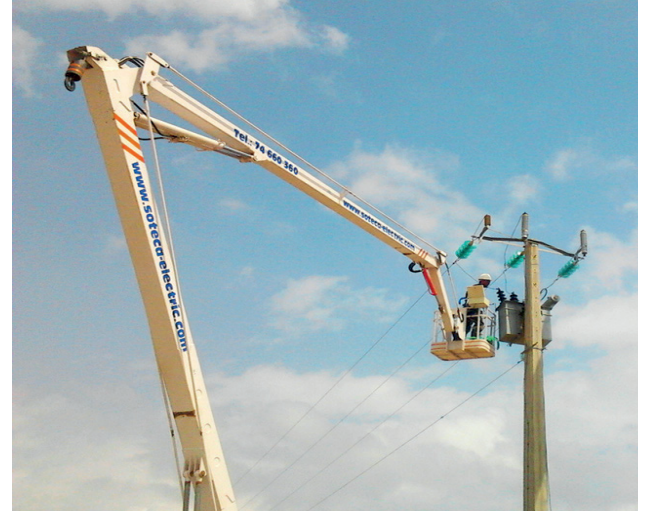
Project: Transformer Station (Kerkennah, Sfax - Tunisia) Client: Serept
