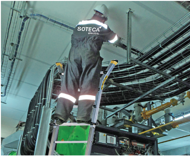
Project: Cogeneration (Sousse - Tunisia)
