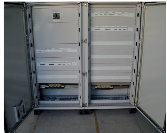
Project: Export of electrical panels (Mauritania) Client: SNIM
