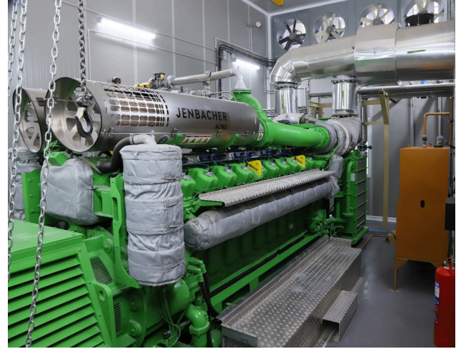
Project: Cogeneration (Sfax - Tunisia) Client: STPA
